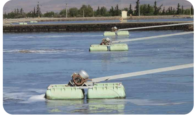
OxyStar® Aerators in Operation
