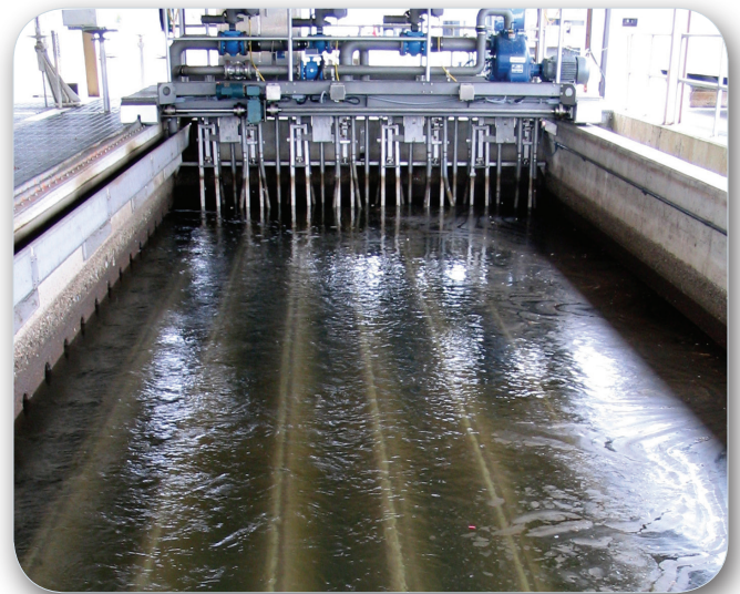
One of the AquaDiamond® filters retrofitted into an existing traveling bridge filter tank at Little Falls Run.
