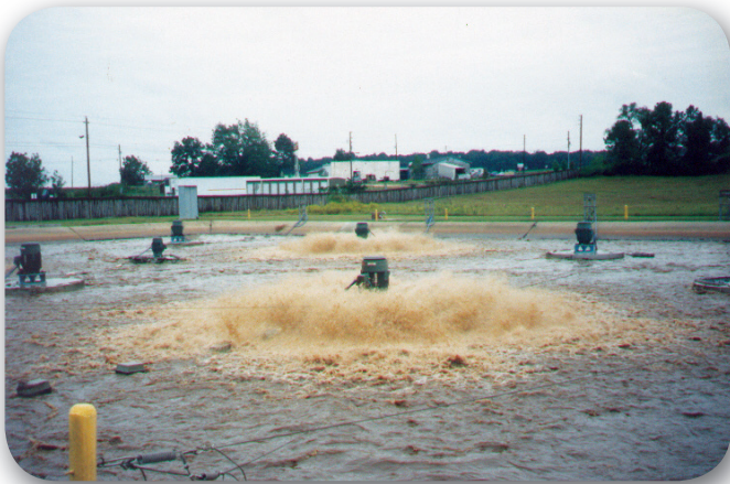
One of the AquaSBR® basins in operation at Birds Eye Foods. Shown are the Aqua-Jet® aerators in operation and an AquaDDM® mixer to the left.
