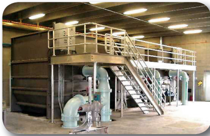
AquaDisk® filters reside inside Tertiary Treatment Building.
