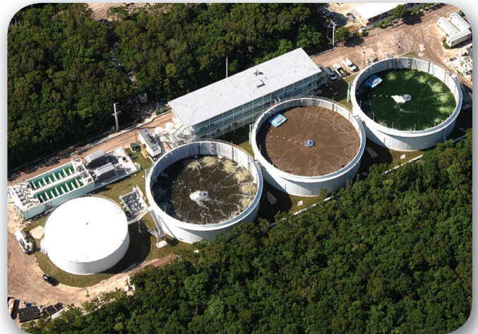
Aerial of Key Largo WWTD after its upgrade with the AquaSBR ® system, AquaDisk ® filters and IntelliPro ® system.
