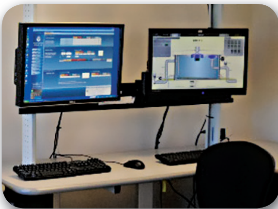
IntelliPro® monitor (shown left) is displaying AquaSBR® basin status at Key Largo WWTD
