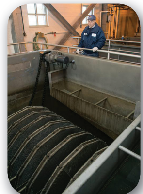
Superintendent, Alan Zerbato visually inspects one of the AquaDisk filter units. © 2014 Ed Collier Photography
