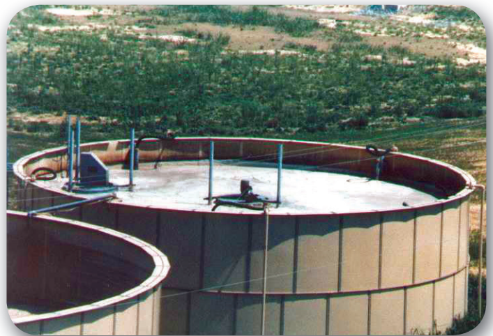
Single basin AquaSBR ® system measures 47' in diameter x 16' SWD.
