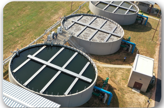
AquaNereda ® Reactors Riviera Utilities Wastewater Treatment Plant at Wolf Creek – Foley, AL
