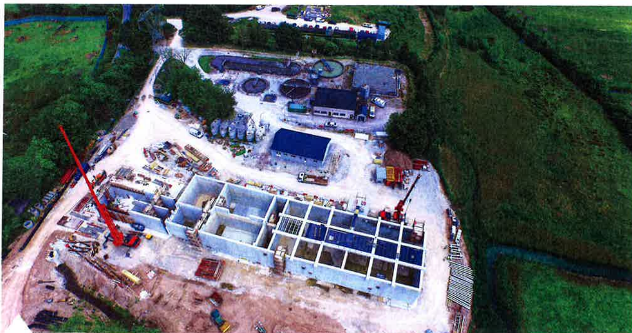
Carrigtwohill Wastewater Treatment Plant
