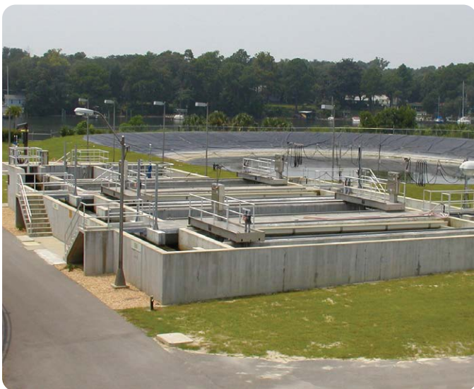
Four AquaABF ® concrete filters installed as part of this plant's upgrade to meet required effluent TSS and phosphorus levels.
