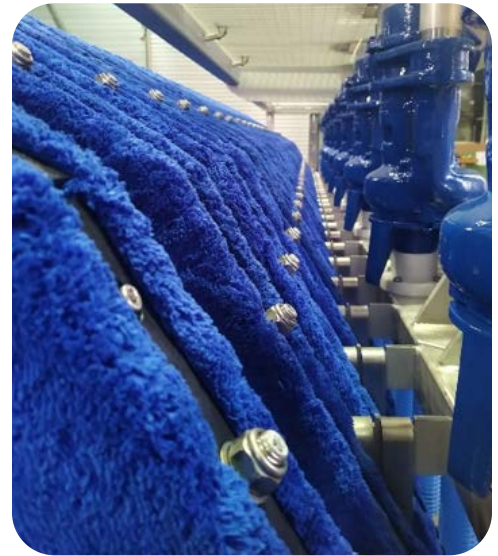
Internal backwash pumps and OptiFiber® Cloth Filtration Media mounted on preassembled frames
