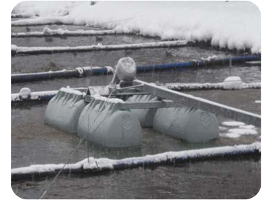
TurboStar® in activated sludge basin
