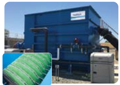
Linda County Water District, Olivehurst, CA
