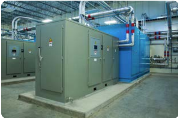
Power Supply Units
