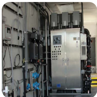
Controls and monitoring equipment
