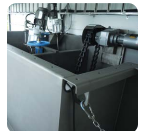
External view of the compact filter tank using OptiFiber® pile cloth media.
