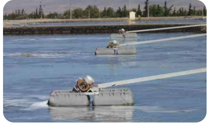
OxyStar® Aerators in Morocco - Aerated Lagoon
