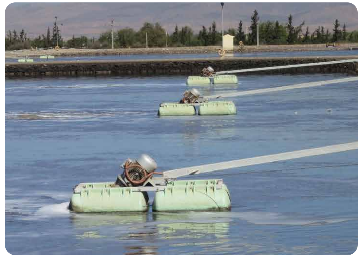
OxyStar® Aerators in Operation
