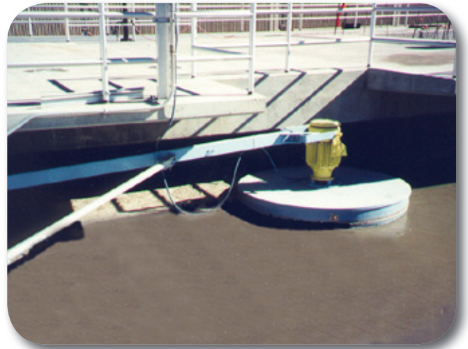
This AquaDDM ® mixer with a pivotal mooring arm can be pulled to the port for ease of maintenance.
