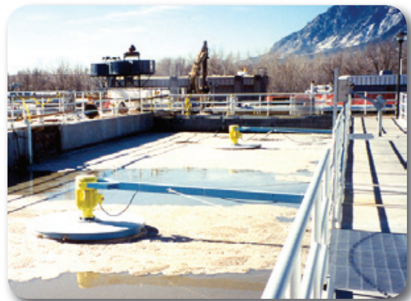
One of five anoxic basins utilizing AquaDDM® mixers with a pivotal mooring arm.
