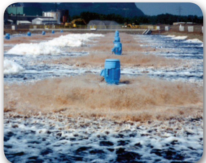
A number of MacLaren's Aqua-Jet ® aerators in operation. The ThermoFlo ® spray coolers can be seen in the background.
