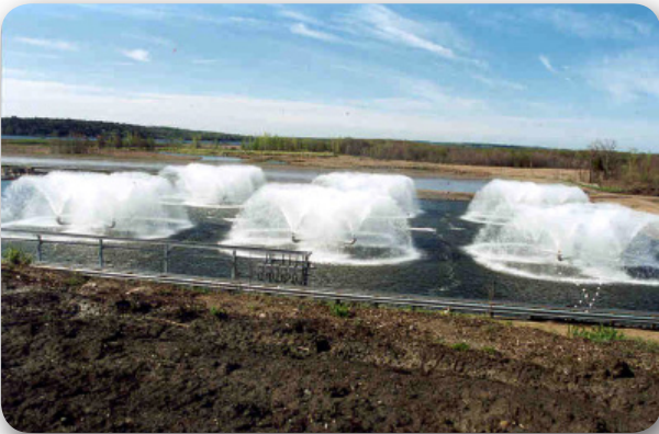
ThermoFlo® Spray Coolers in operation.
