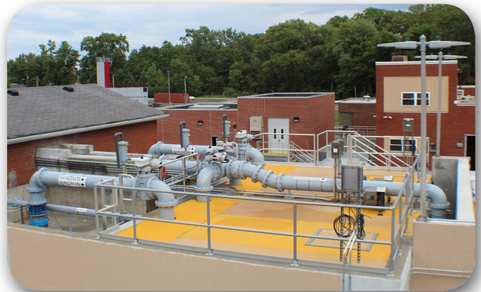
Covered AquaPrime® cloth media filters were retrofitted into the abandoned sand media filter structures.
