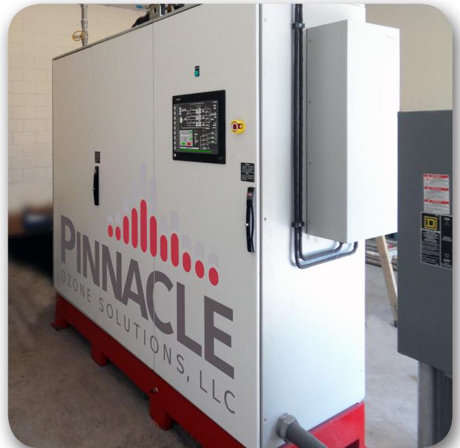
Pinnacle M-Series 30x ozone system selected by the City of Sanford, FL for the WTP facility.
