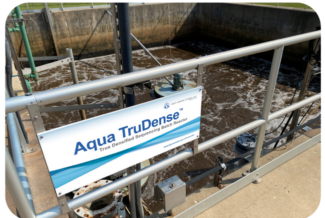
All Phases of Treatment in a Single Basin
